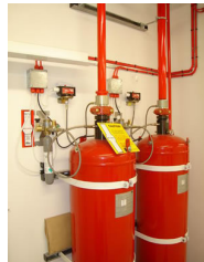
Gas suppression system
